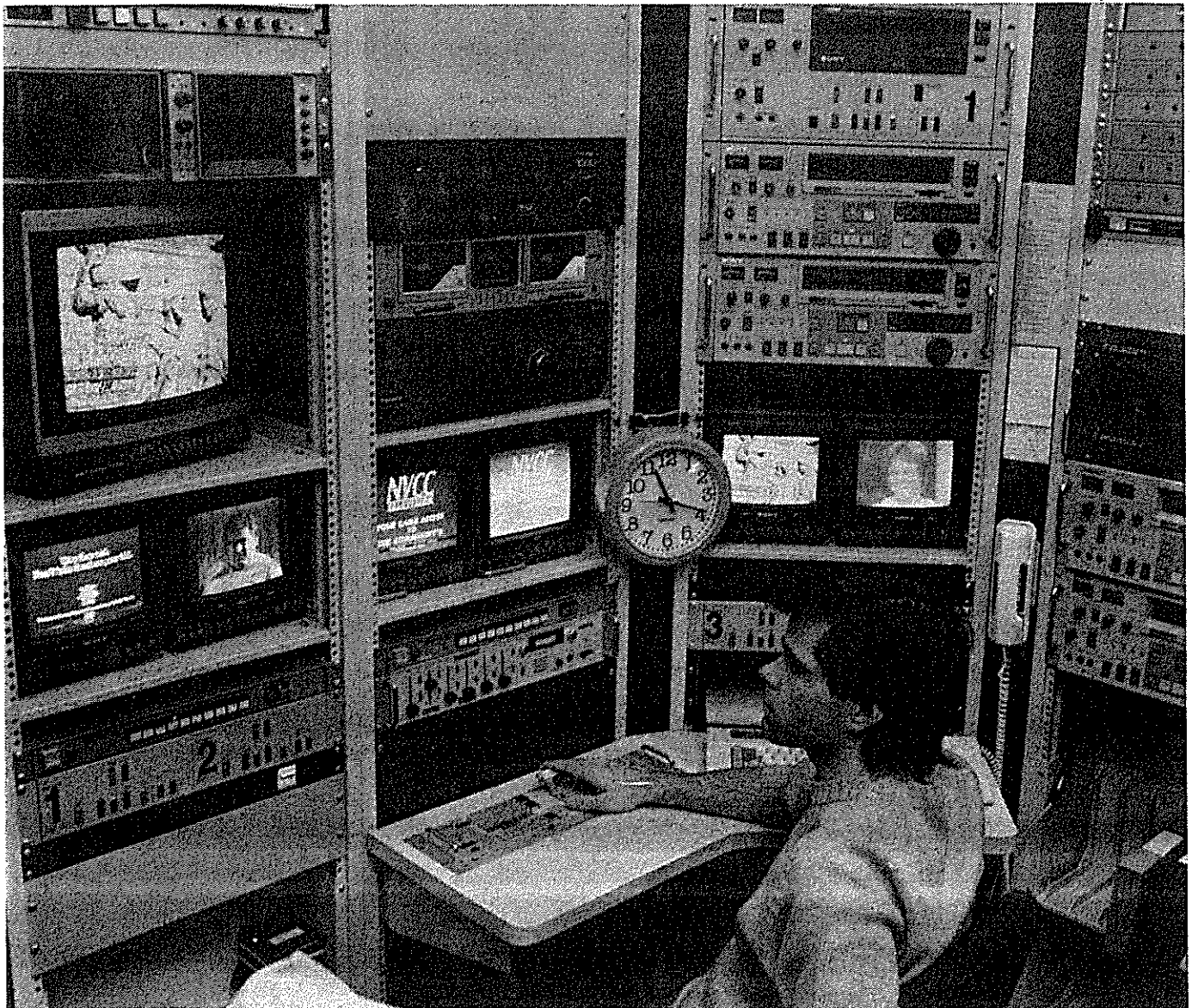
Telecommunications Control Room
